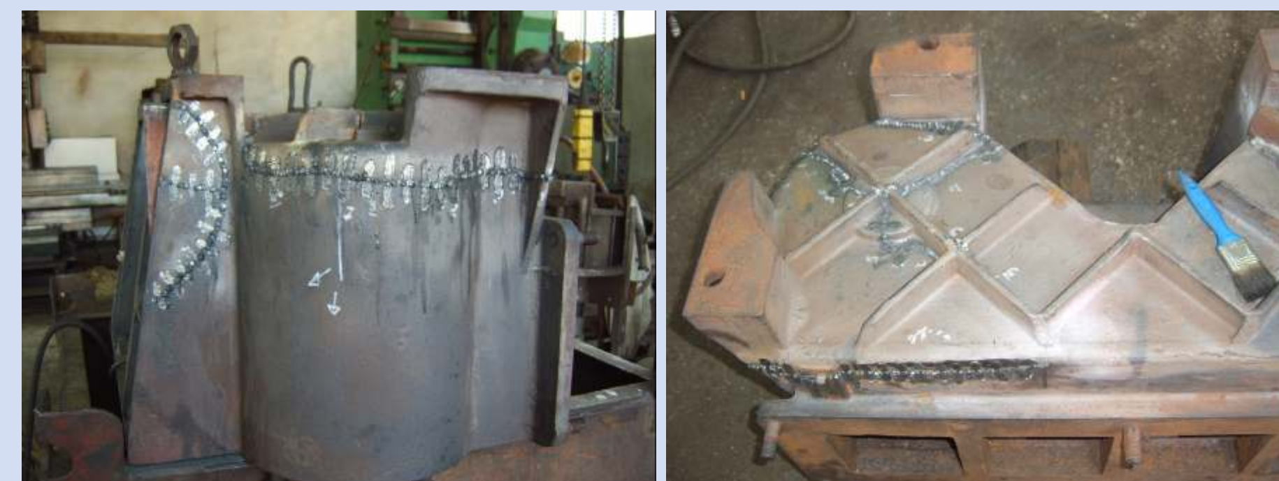
Stages of the Metallock repair of the piston pump casing (fig.3 and 4)
