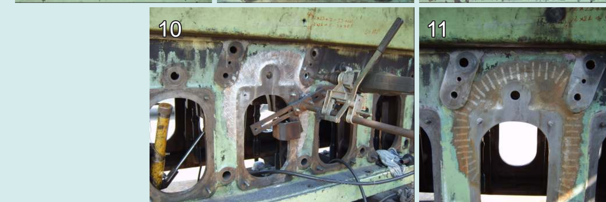
Final repair works and completed METALOCK repair of external left wall (fig.10, 11)
